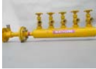
Acetylene Manifold with dry type flash back arrestor / Pipelines – Service brown band on canary yellow
