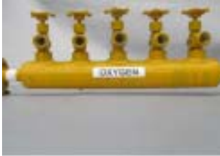
Oxygen Manifold/Pipe lines – White band on canary yellow
