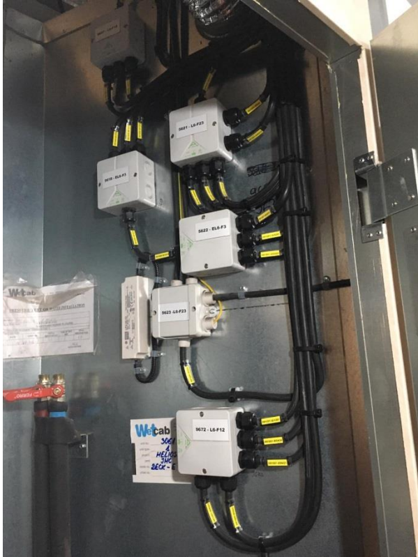
Figure 28: Junction boxes at the rear of a wet cabin
