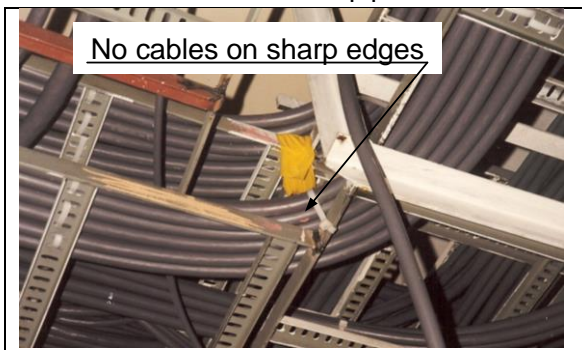
Figure 22: Cables wrong installed on sharp edges
