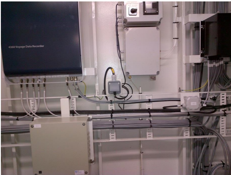
Figure 36 grounding of communication equipment with a gn/ye wire.
