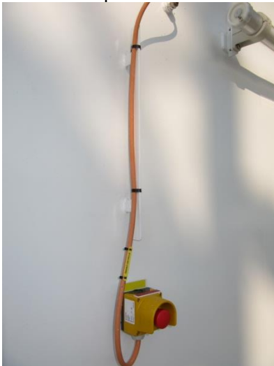
Figure 39 Outside cables NOT preferred
